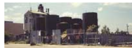
Former Van Iderstine. Tall building is the mill where rendering and processing takes place. Vertical Tanks are storage tanks where finished products, fats, and oils are stored. Triplex Oil would be horizontal green tanks. (Spot 6) per Huneke 1998 Camera looking West Credit: Carl Fabrizio
