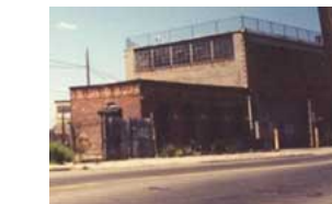
Shaw Walker (Spot 10) on corner of Review Avenue and Laurel Hill Boulevard, sidewalk is a feature that should be modeled July 1998 Credit: Carl Fabrizio
