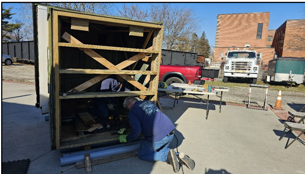
The next step was to build a wood frame to support the floor. Do notice a RMLI volunteer inside of the shanty!
